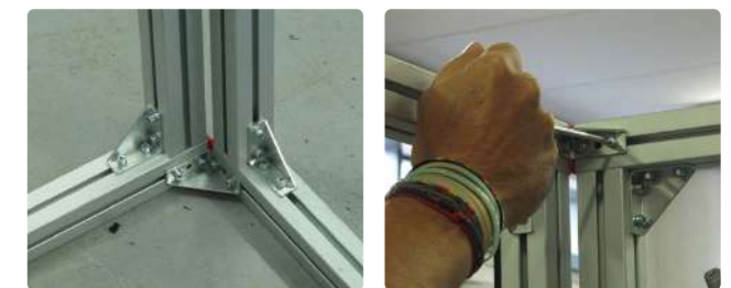
Fix frames with 4 brackets on the top and 4 brackets on the top
